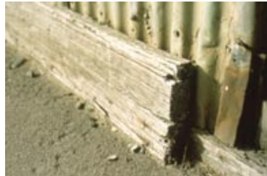
Natural weathering of unprotected plinth (Photo courtesy of Dr. Harry Greaves)
