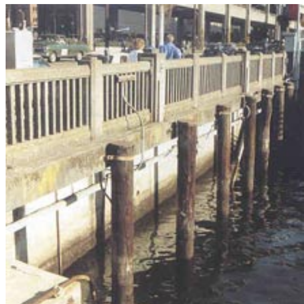
Fender piles require protection against marine borers and need high wear resistance.
