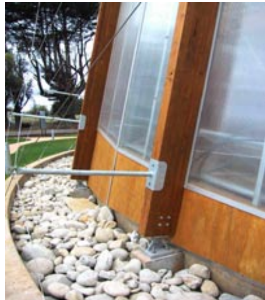
Good detailing of wood-based composites to eliminate water penetration as well as corrosion. (Photo courtesy of Dr. Harry Greaves)
