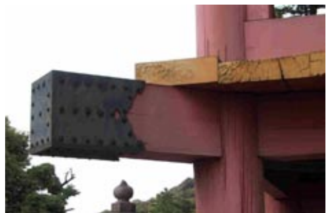
Metal physical shield to protect against water uptake at the most vulnerable point of the structure. (Photo courtesy of Dr. Harry Greaves)
